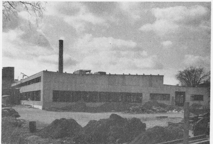
With construction details proceeding according to plan, the Waterville Division's sand casting foundry is expected to be completed in August. The interior is being prepared to receive the latest modern machinery and operations will commence in the early Fall. The foundry will employ 125 in producing castings for several Scovill divisions and plumbing fixtures for small homes.
